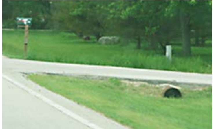
Protruding Drainage Pipe
